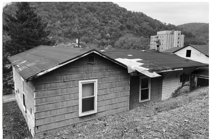
One of the unsafe houses SALS works on to make livable for its owners
