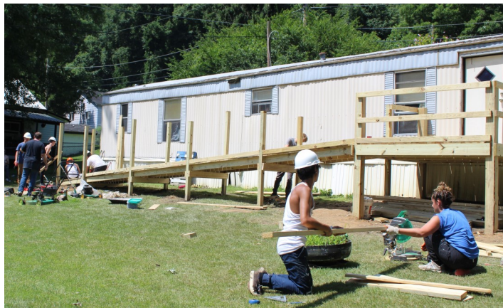
Volunteers work with SALS to construct a wheelchair ramp for a local resident with disabilities
