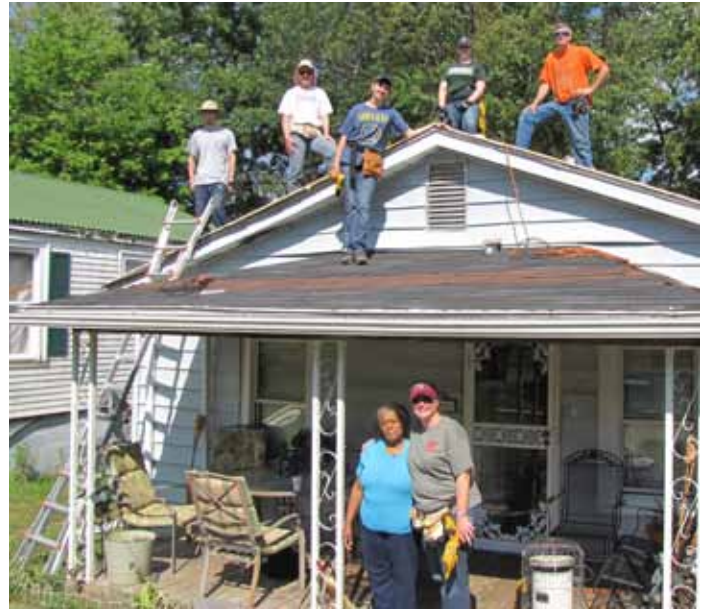
ASP volunteers from Cornwall UMC in New York are putting on a new metal roof for Valerie Waller (on left on porch)
