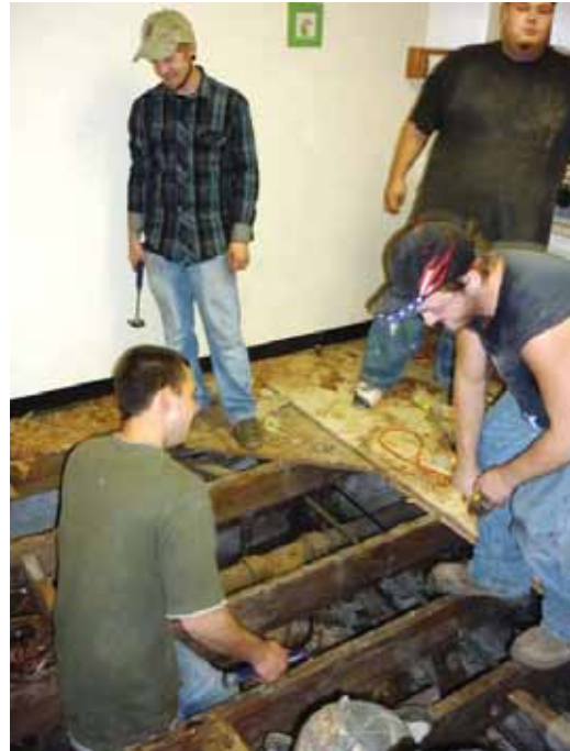
YouthBuild members repair bathroom in Community Center on Make a Difference Day
