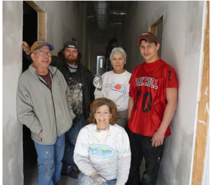
SALS staff and volunteers drywall finishing crew in new volunteer dorm being built at Beards Fork
