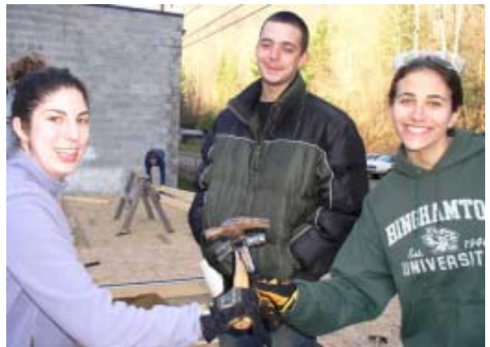
Volunteers cross hammers getting ready to frame the new dorm at SALS Community Center
