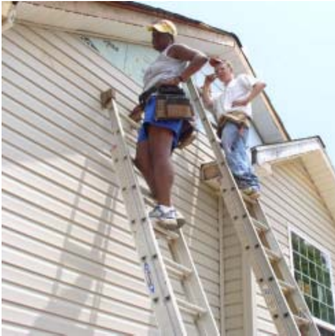
Sam Pozzie and Global Volunteer install siding on a house at Sids Lane
