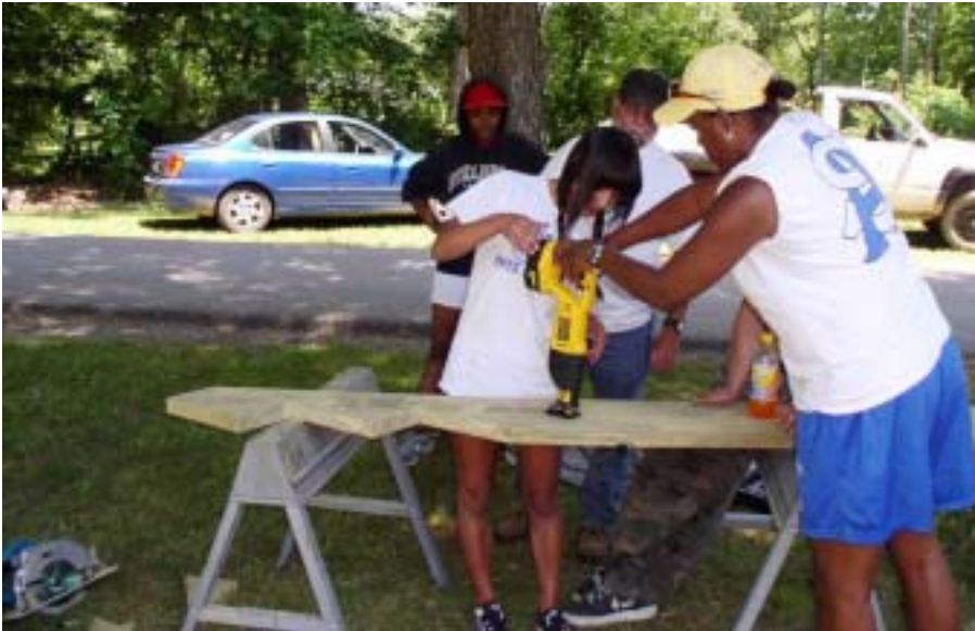
Dave Shaver watches as volunteers learn how to use a reciprocating saw to cut stair risers
