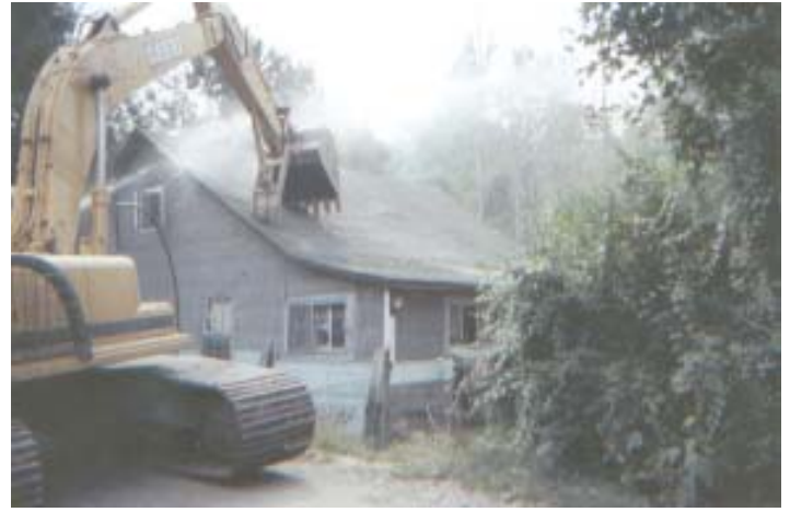
Out with the old: backhoe demolishes dilapidated home to make way for new construction in Page
